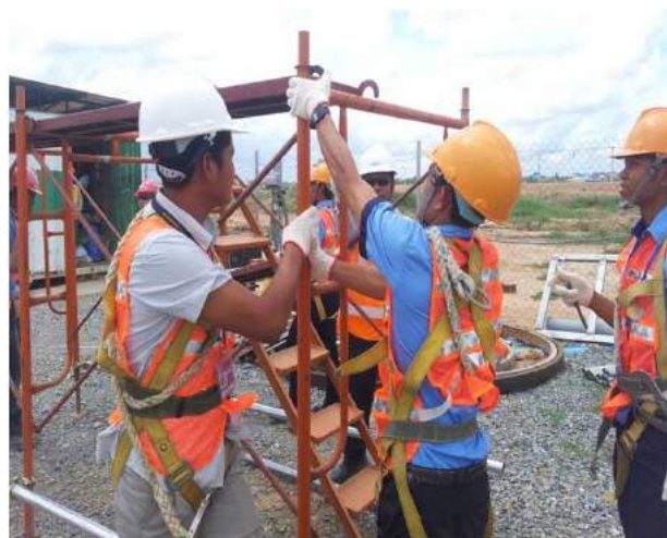
Training in assembling scaffolding, offered by the Vinci Construction Company Grands Projets
